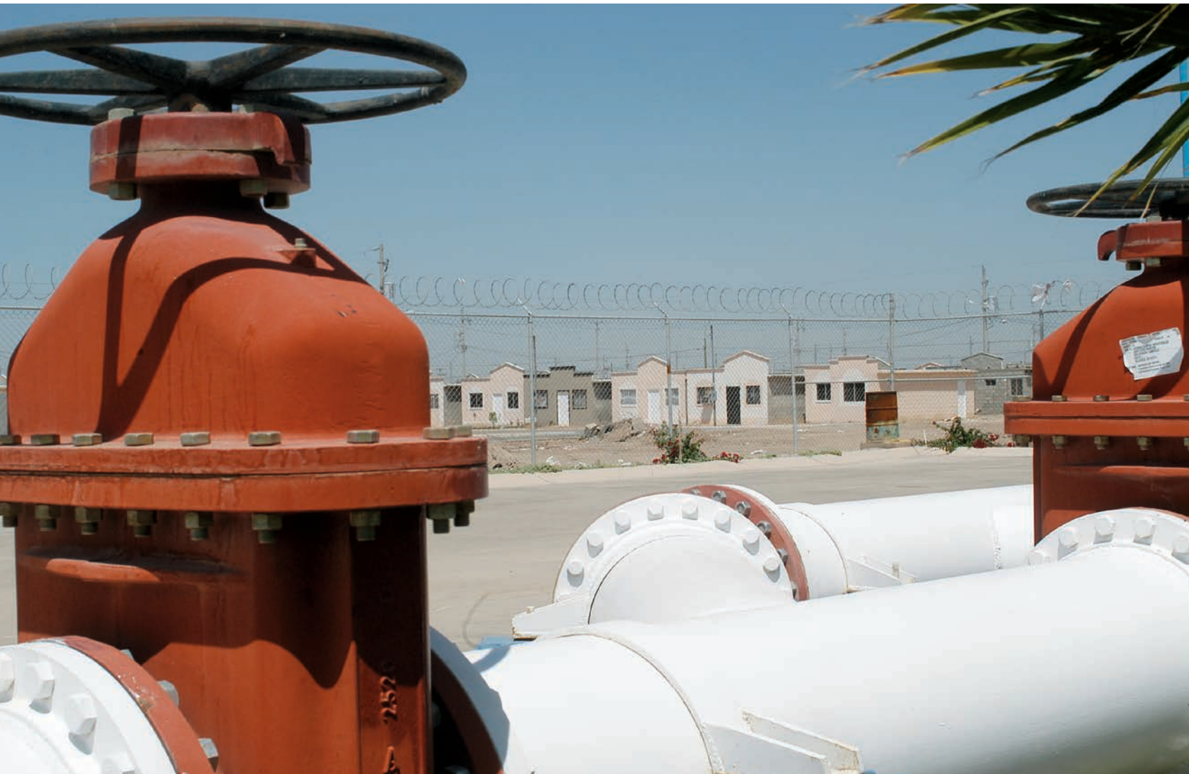
Wastewater Pump Station PB6 was constructed with NADB funds under the Sanitation Program in Mexicali, Baja California. In addition to providing improved service to current customers, new housing development has been possible because of this project. (Certified: December 1997 / Completed: September 2007)
