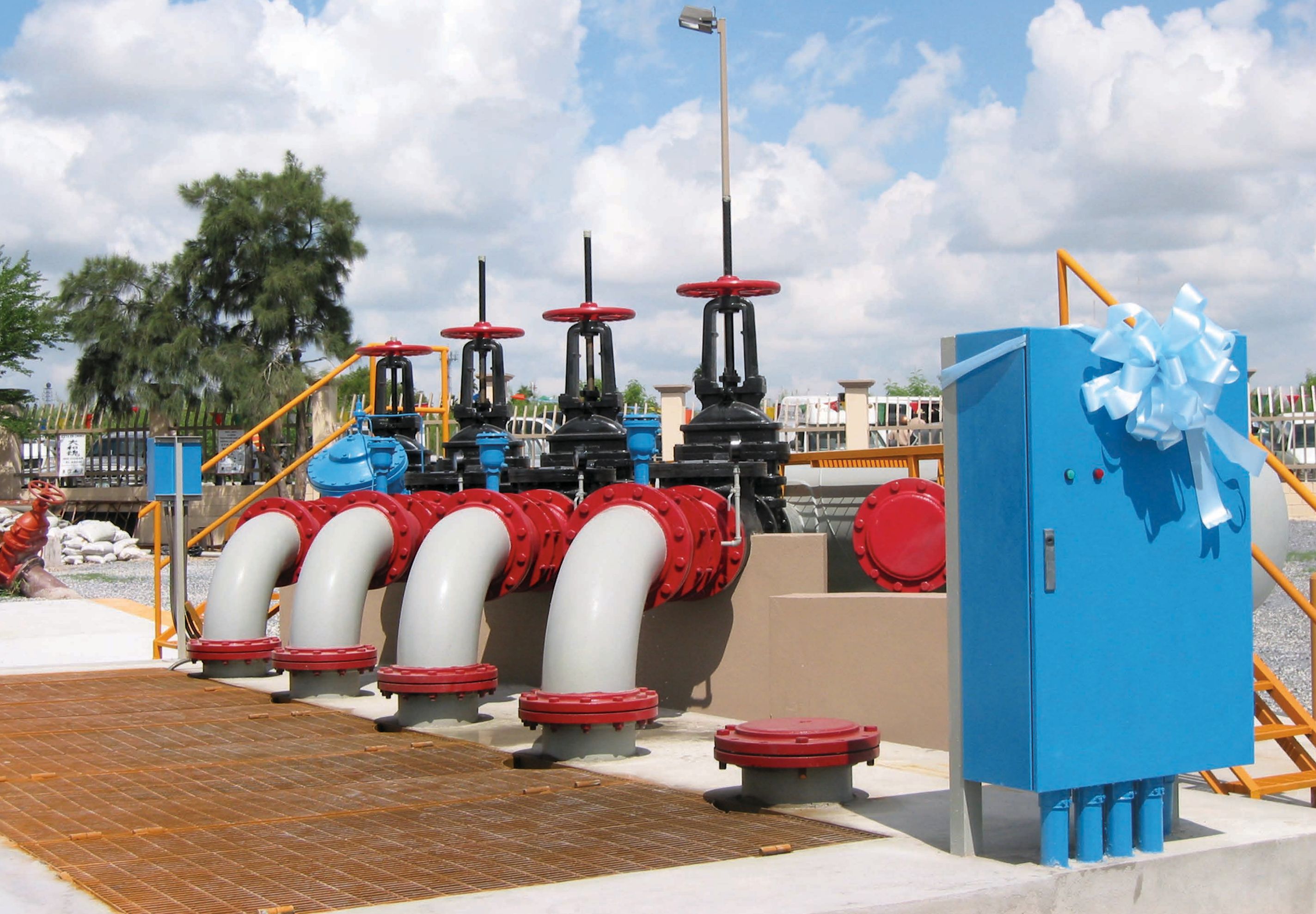
Pump Station No. 10 with the capacity to pump 38.8 million gallons a day of wastewater began operations in 2003 and was an important component of the Comprehensive Sanitation Project in Reynosa, Tamaulipas. (Certified: March 1998 / Completed: May 2011)
