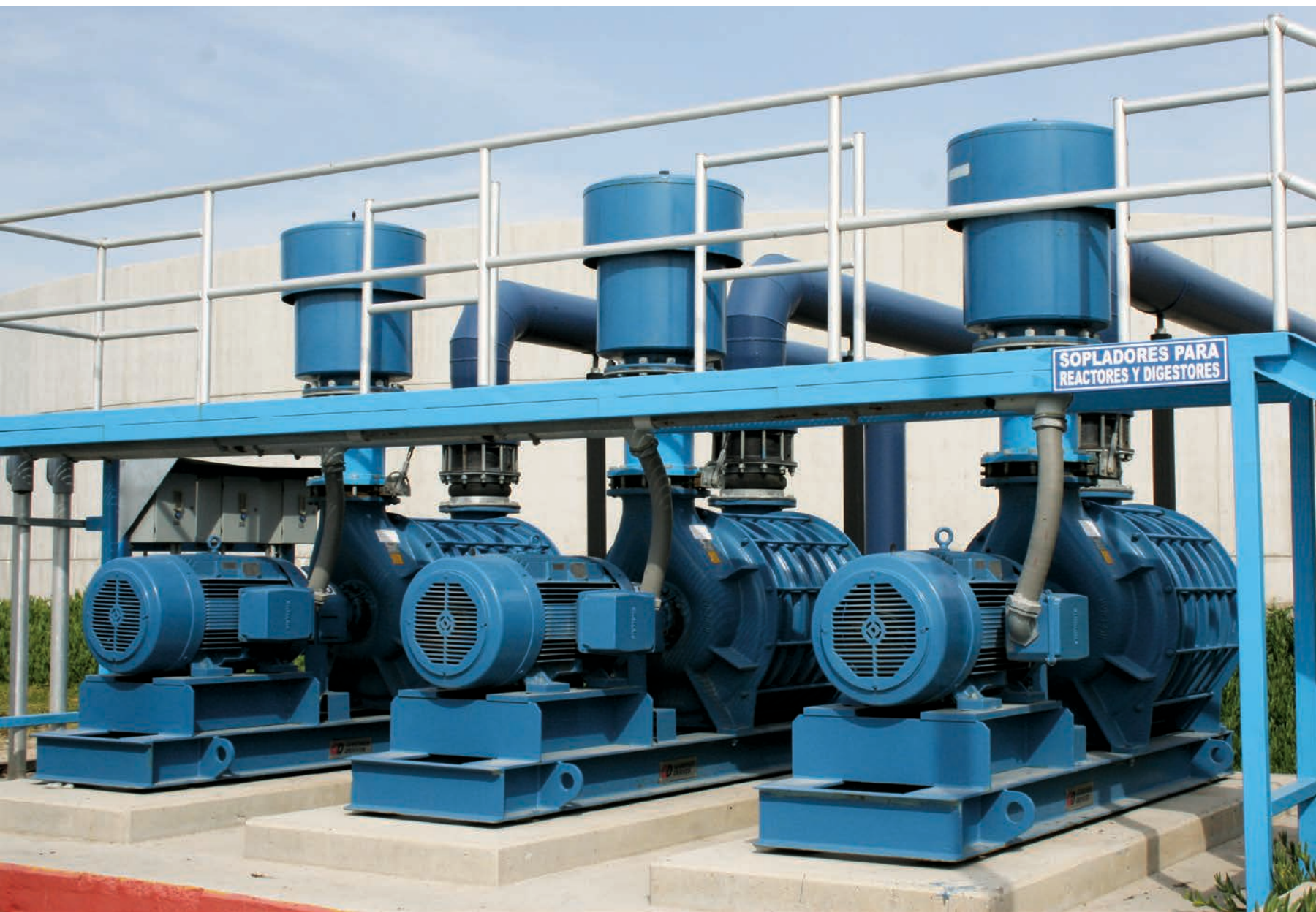
The La Morita Wastewater Treatment Plant in Tijuana, Baja California, can treat up to 5.8 million gallons a day of wastewater and is one of seven plants certified by BECC and financed by NADB in Baja California. (Certified: February 2011 / Completed: August 2010)
