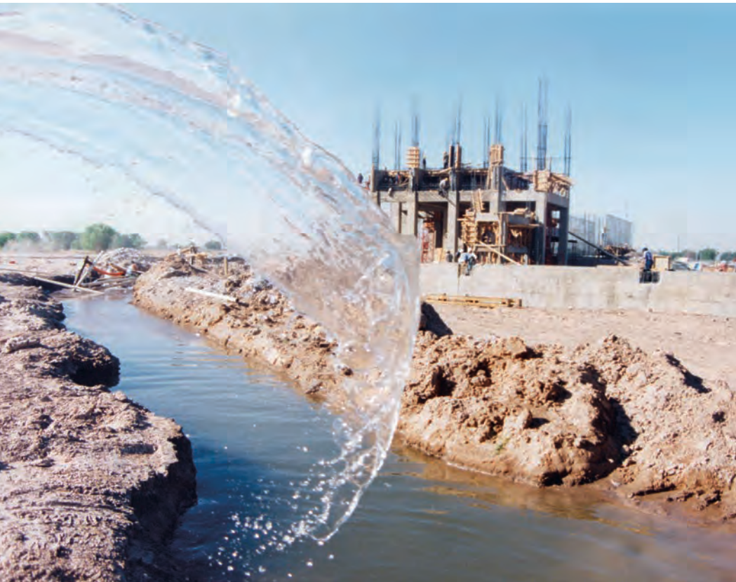
North Wastewater Treatment Plant in Ciudad Juarez, Chihuahua. (Certified: September 1997 / Completed: April 2001)
